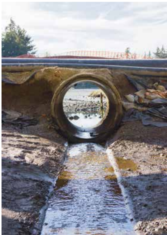
Left: An undersized culvert blocks fish passage in the Carpenter Creek estuary. Below: The Suquamish Tribe and U.S. Navy have partnered to build a bridge to replace the culvert and restore tidal flow to 6,000 feet of estuary.
